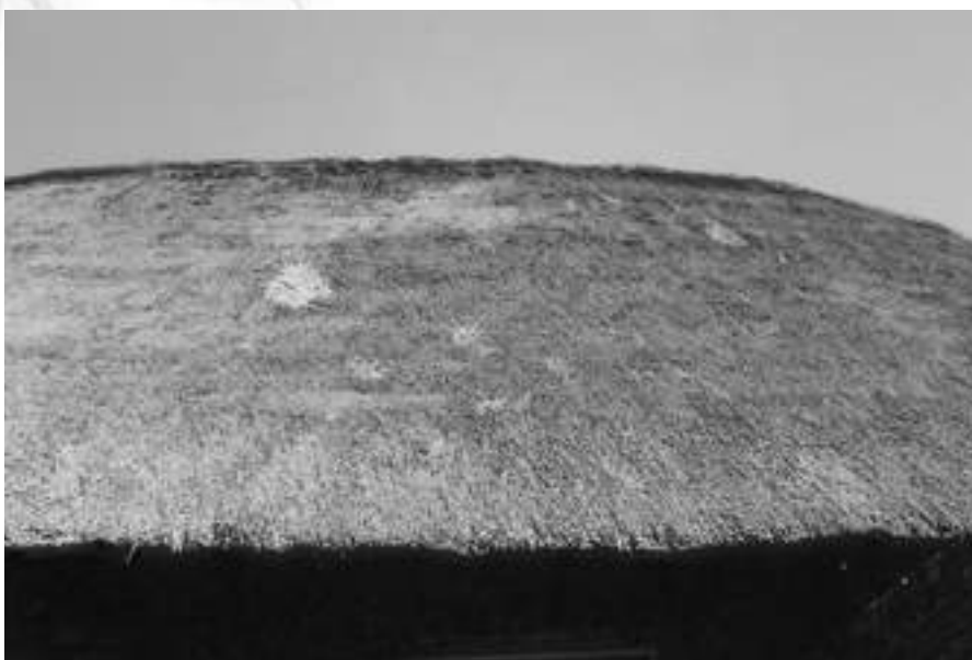
Photograph 9 Typical thatch decay in need of maintenance
